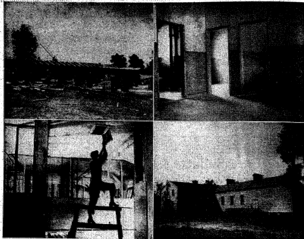
WHAT A LITTLE ENGINUITY AND IMAGINATION CAN DO . . . Reconstruction of unused buildings in the Hampton Church hospital area is under full swing as evidenced by the pictures above. The photograph at the upper left shows a construction gang, under the direction 2nd Lt. Gerald R. Marcus, demolishing an old building. The material salvaged from the old buildings is being used in the renovation of other buildings in the area. In the foreground may be seen the foundations of an already demolished structure. In the photograph at the lower left electrical connections are being installed in a half completed unit. Plywood wall paneling has been erected and awaits in place. To the upper right the nearly completed apartment is shown with well planned corridors and surrounding area. The apartment is shown with well planned corridors and surrounding area. The apartment is shown with well planned corridors and surrounding area.
